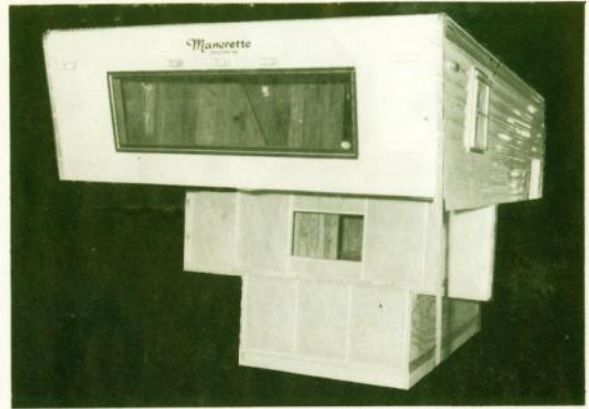
Pictured above. A basic camper model during construction. Shown is a good example of careful construction and generous insulation.
